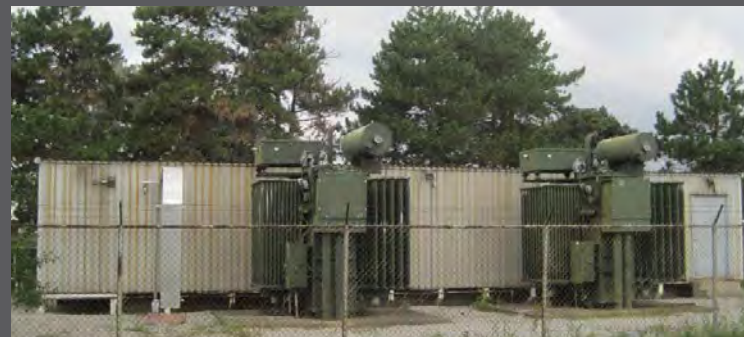
Wastewater Treatment Plant Substation (Constructed early 70's)
