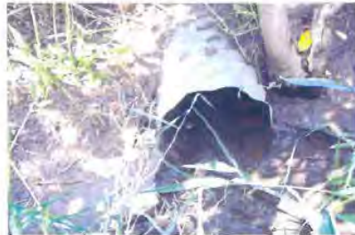
Partially Full CSP
