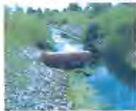
Corroded CSP from QEW Median
