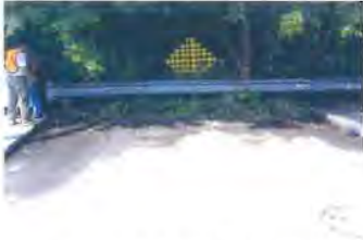
Build-Up of Debris
