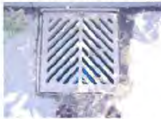
Catch basin Full of Water and Debris
