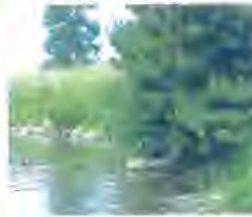
Outlet of 1600 mm \phi CSP Into Red Hill Creek
