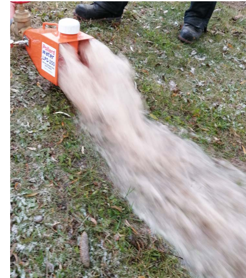
Flushwater flowing out of a diffuser connected to the flushing hydrant with a hose
