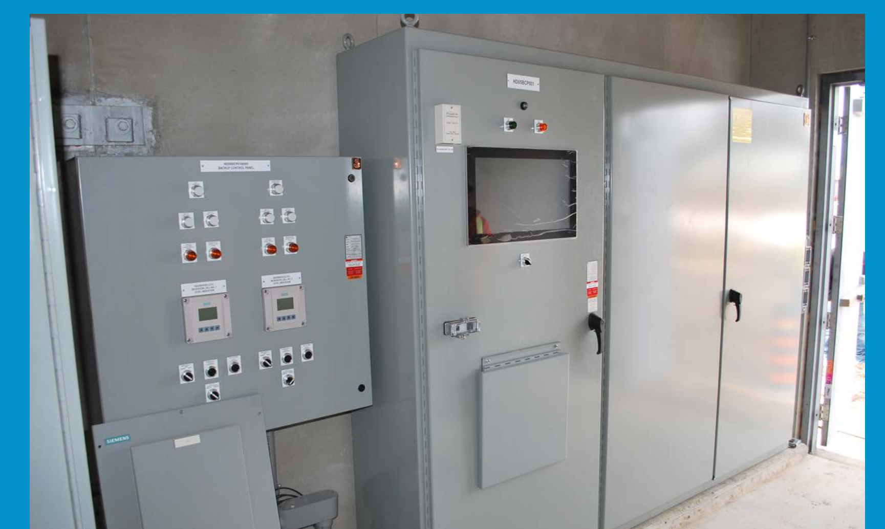
Primary and backup control units
