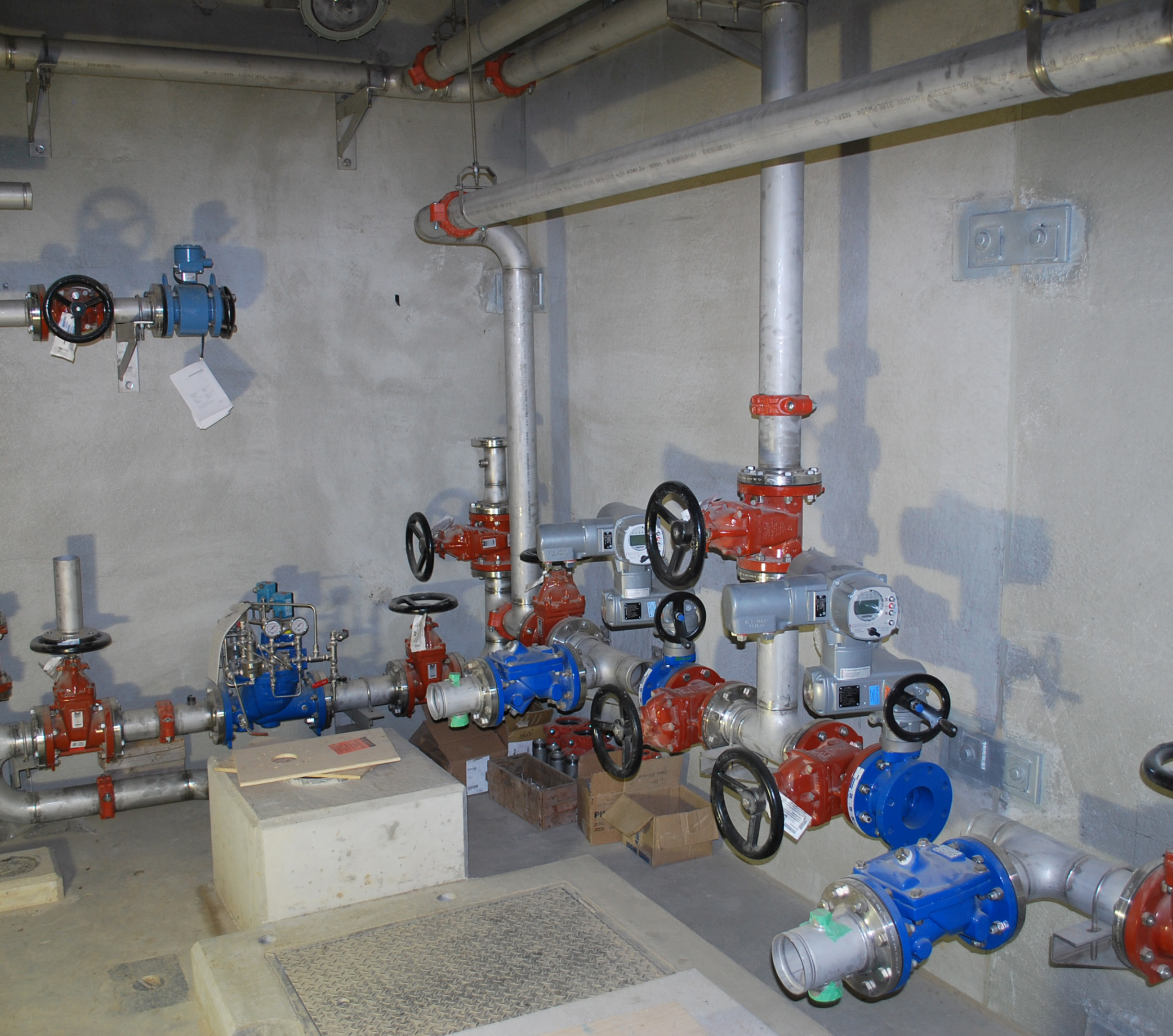
Piping and valves for high lift pumps
