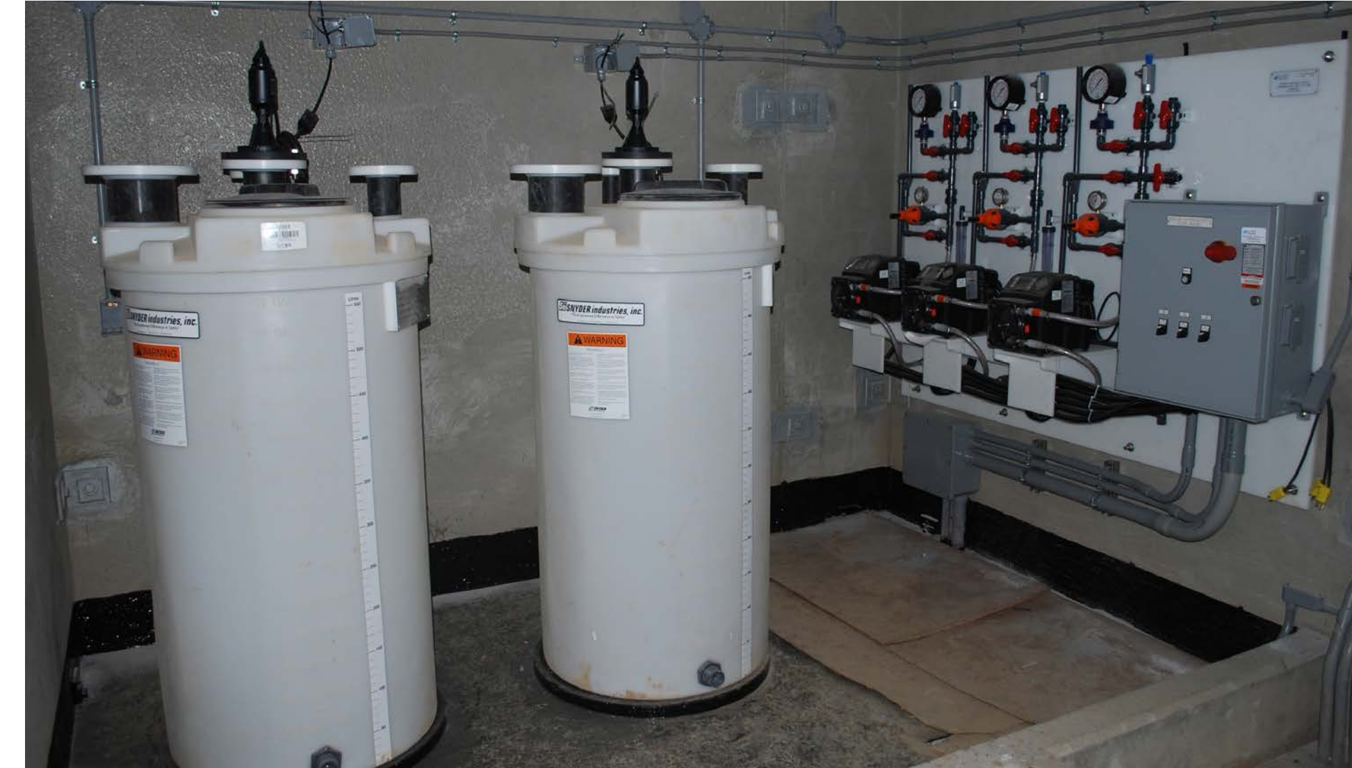
Hypochlorite disinfection storage tanks and chemical pumps
