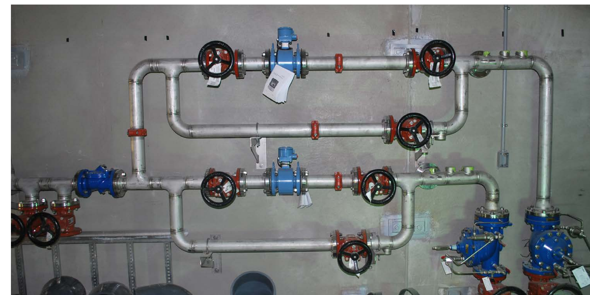
Piping and valves for municipal wells
