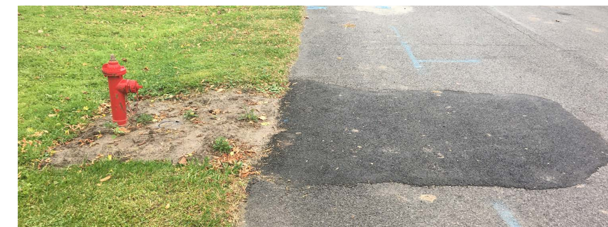
A recent flushing post hydrant installation
