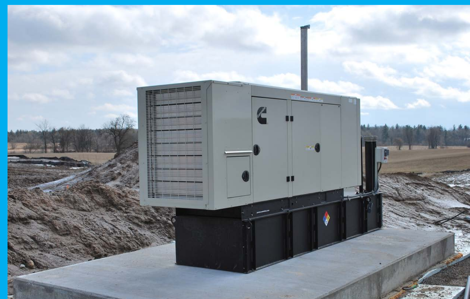
New backup diesel generator
