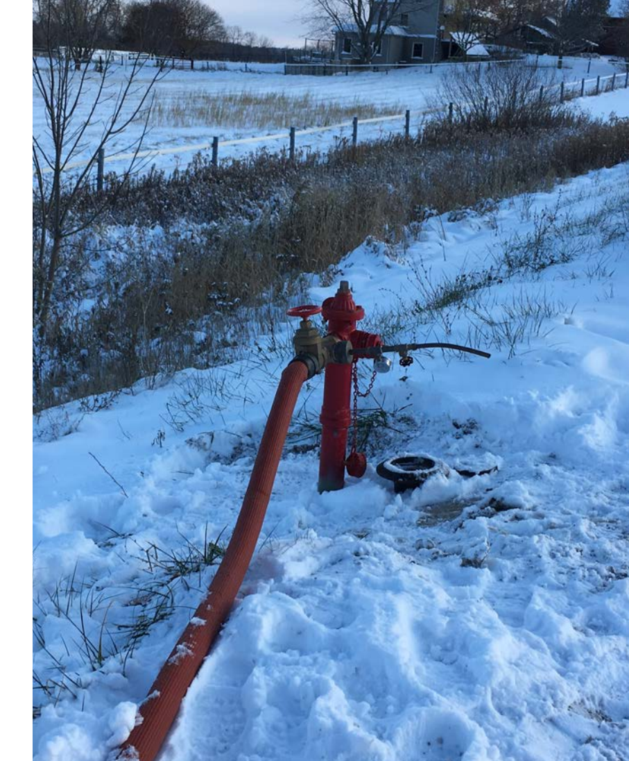
Flushing hydrant with sampling port and hose
